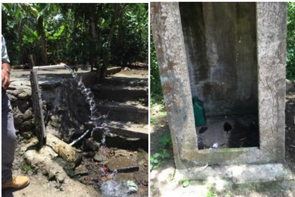
The photo on the left shows potable water at the plantation of Angel Galume-president of the Azua center. The photo on the right shows a toilet provided for men and women in Los Cacaos, where seven people were working.
